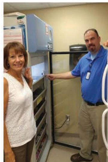
Barb Parker, SCCF advisory board member, and Ted Gaunt, Information Technology Specialist, Story County Medical Center, examine the new power backup system funded by a $2,141 SCCF grant for the Zearing Medical Clinic.
